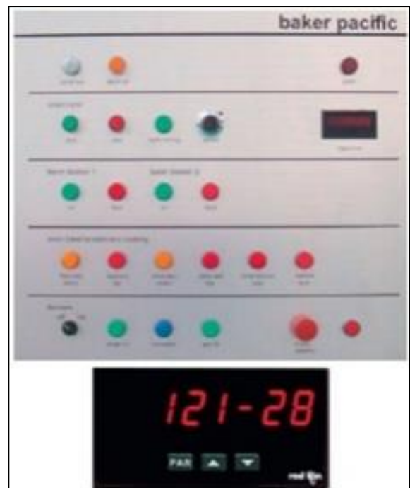
Fig 7: The PAX Lite Process Time indicator from Red Lion Controls is located on the main control panel.
